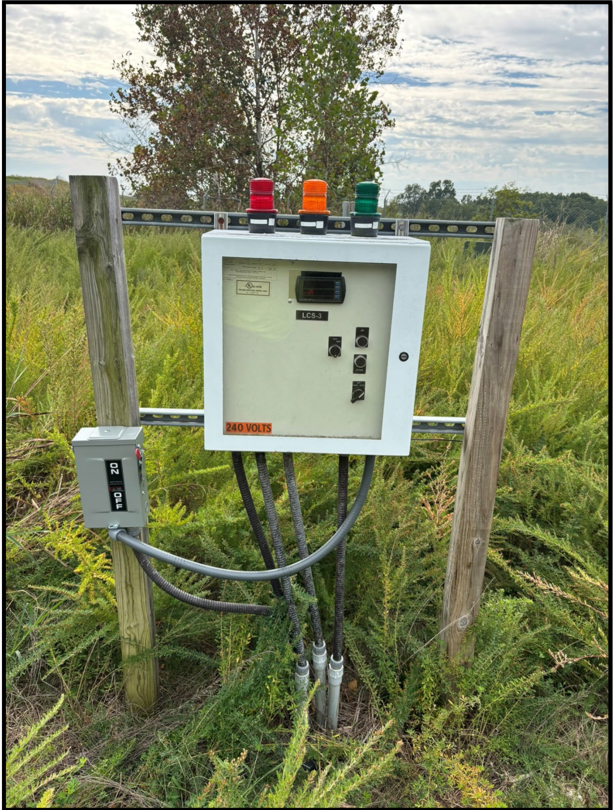
Photograph 3: View of control panel at LCS-3.
