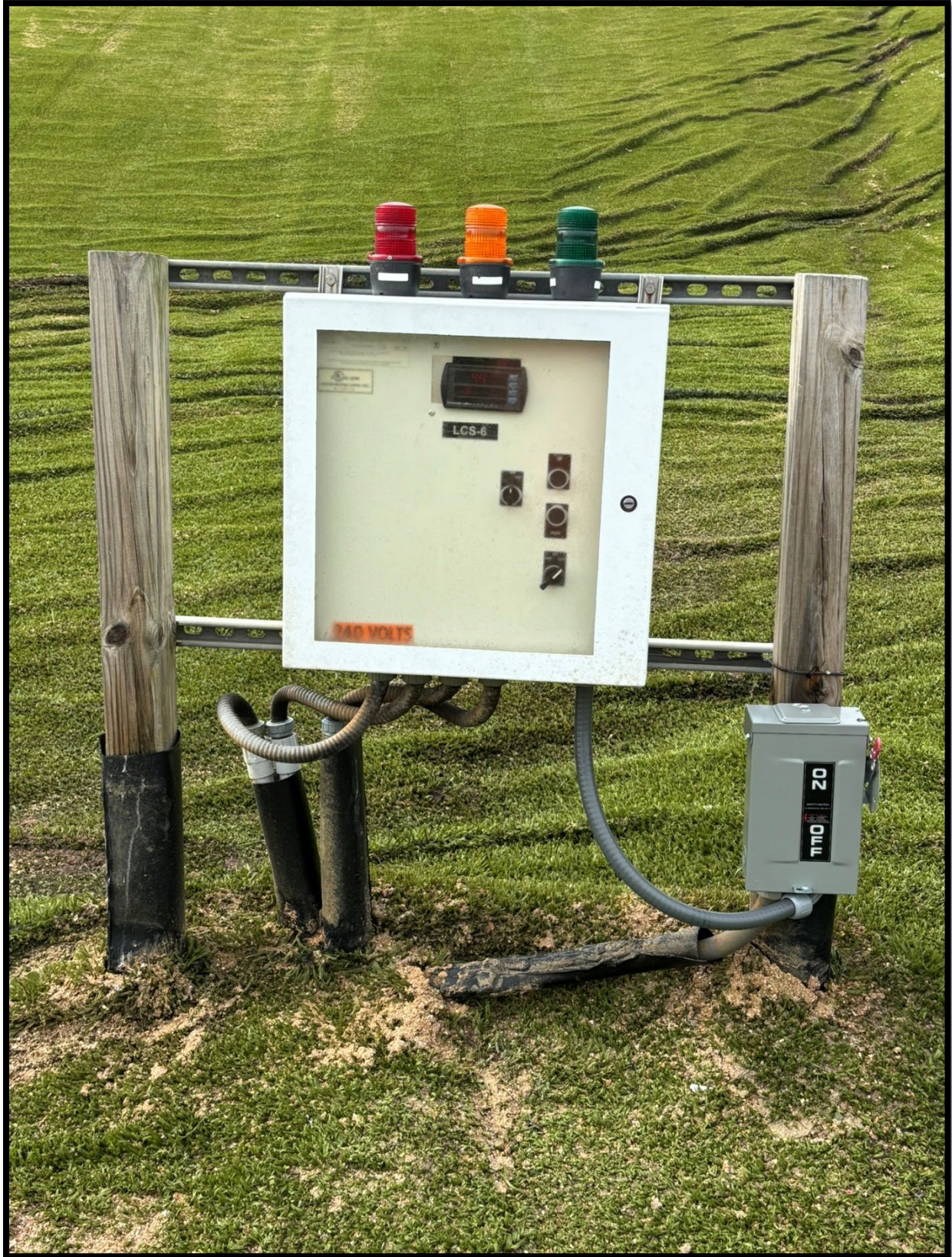
Photograph 6: View of control panel at LCS-6.
