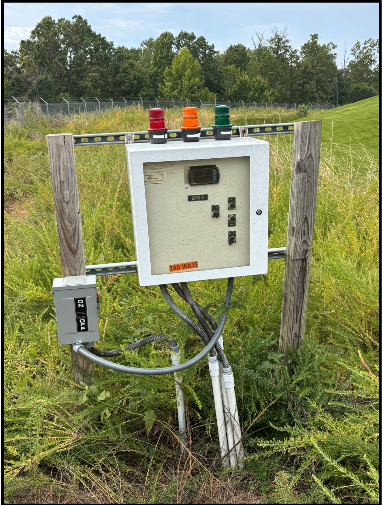
Photograph 2: View of control panel at LCS-2.
