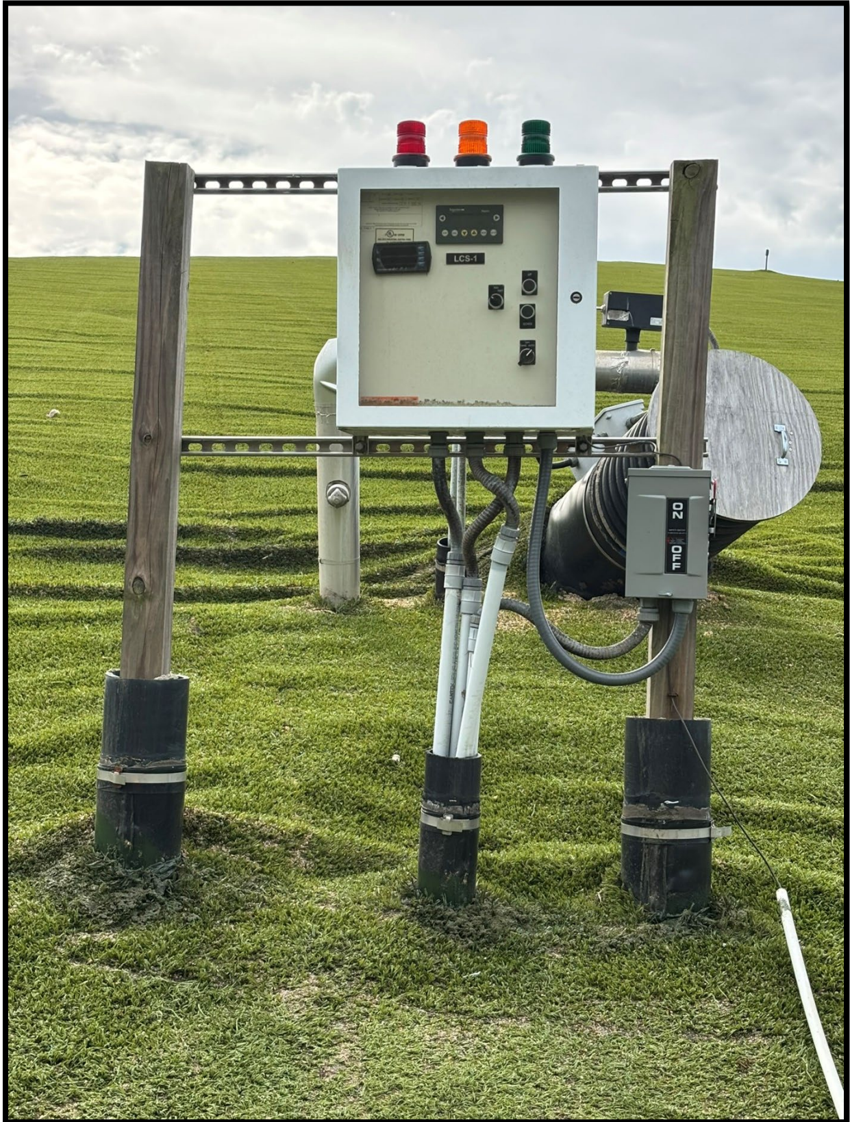
Photograph 1: View of control panel at LCS-1.
