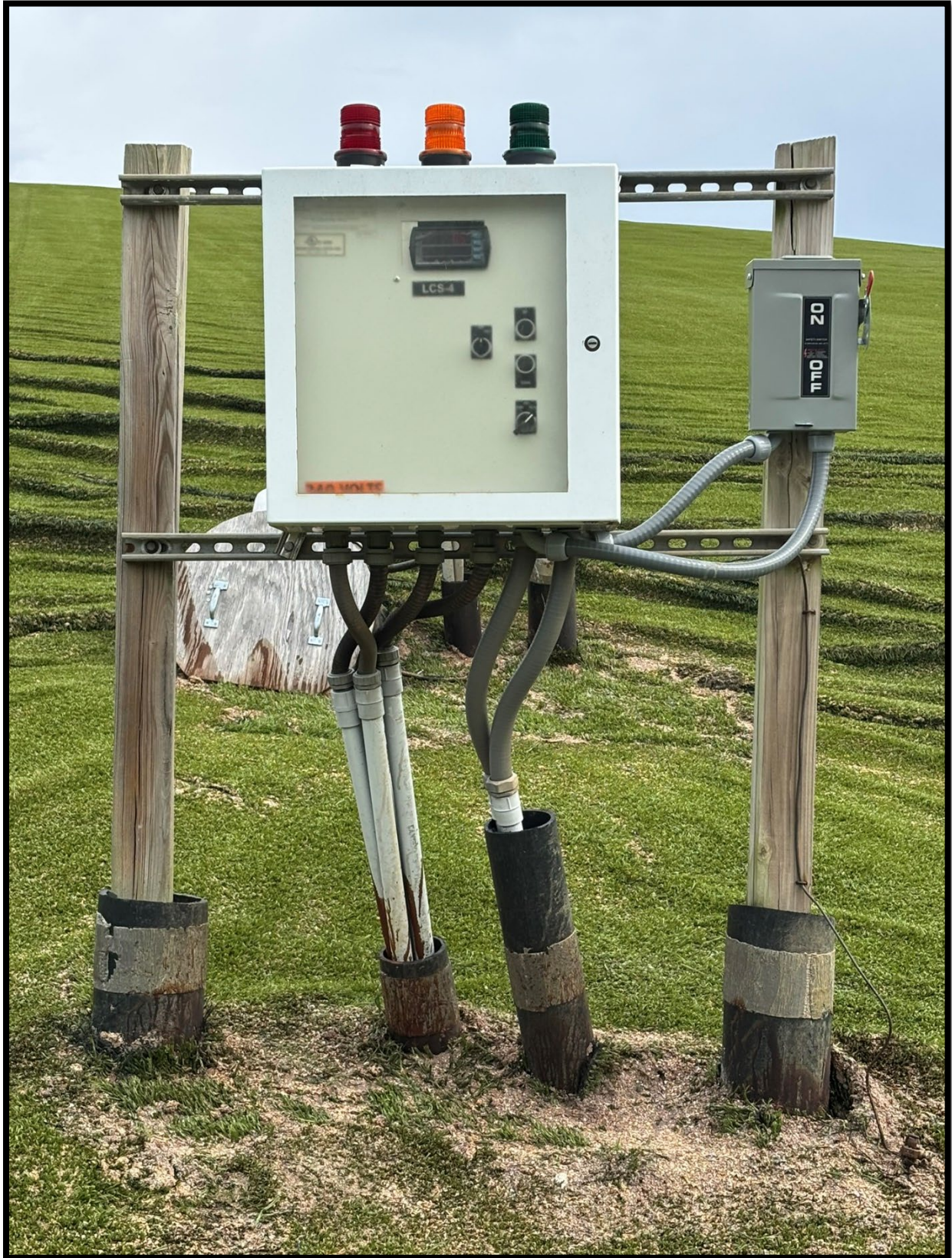
Photograph 4: View of control panel at LCS-4.
