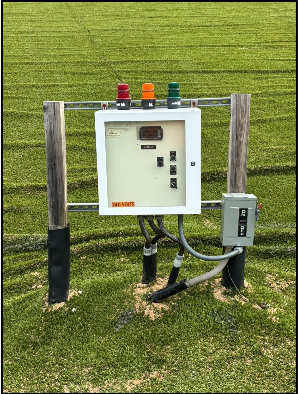
Photograph 5: View of control panel at LCS-5.
