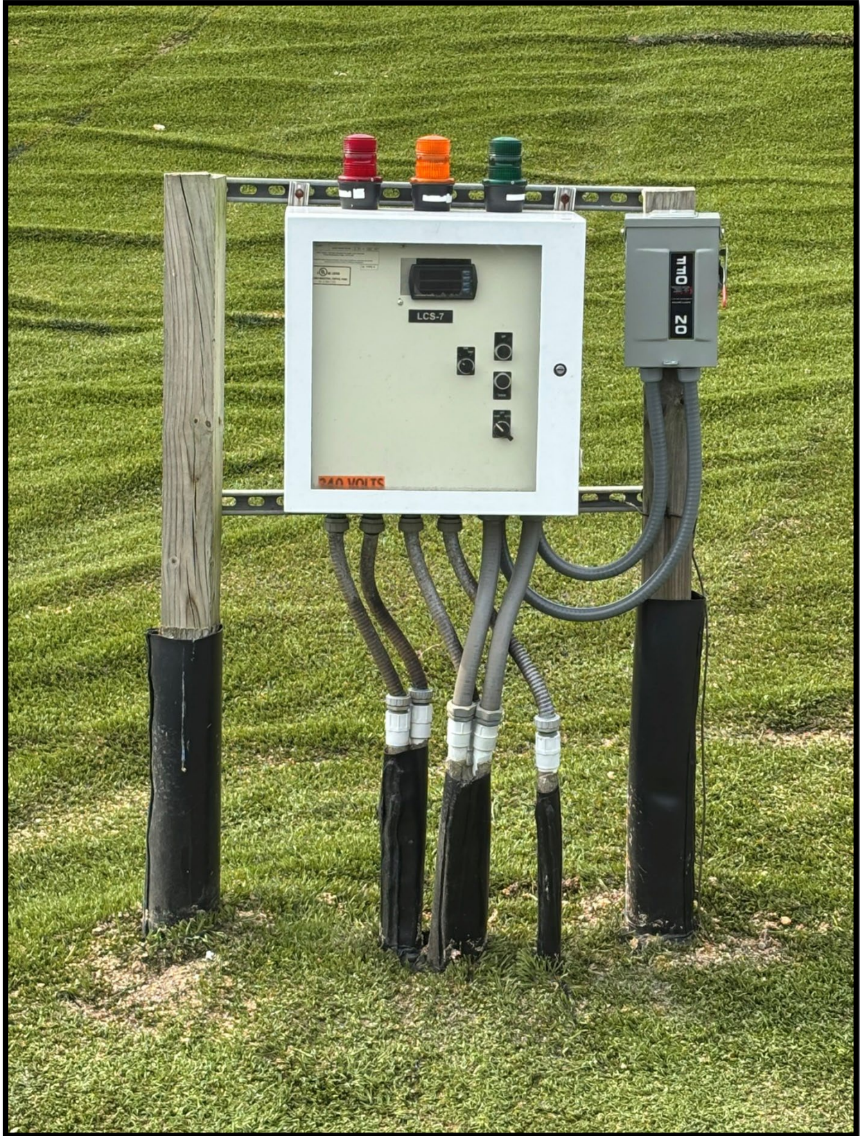
Photograph 7: View of control panel at LCS-7.
